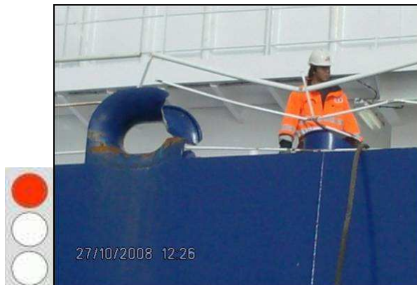
No reinforcement at all!
