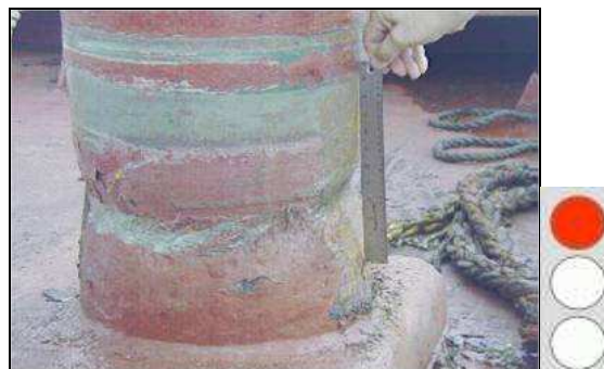
Bitt post crushed due to concentrated load
