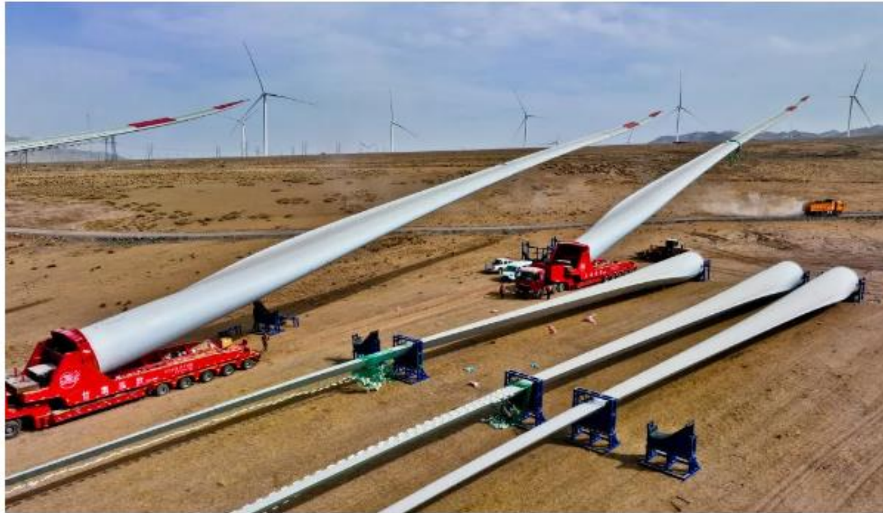
Builders transfer wind turbine blades to a hoisting site at the construction site of a 49.5-megawatt wind farm project in Zhangye, China on March 27. CFOTO/Future Publishing via Getty Images
